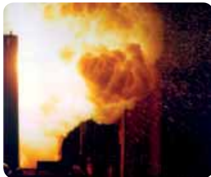
Switchgear explosion due to arc fault
